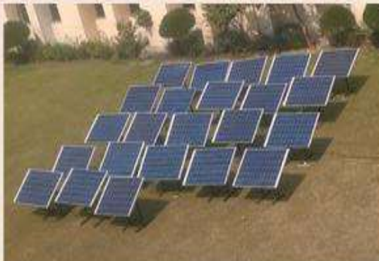
Solar PV Panels
